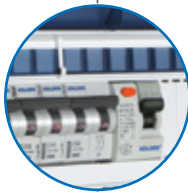
Provision for circuit labeling
